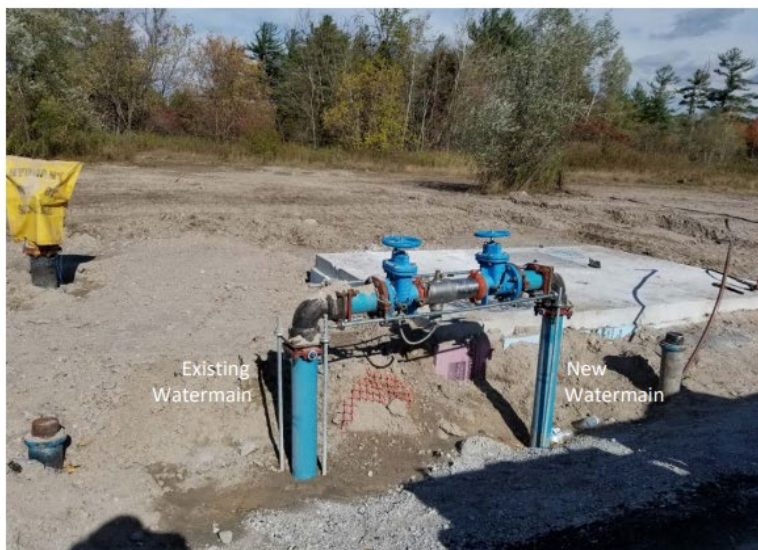
Figure A-2: Temporary connection from a watermain with Backflow Prevention using a CSA-certified reduced pressure principle backflow preventer.
